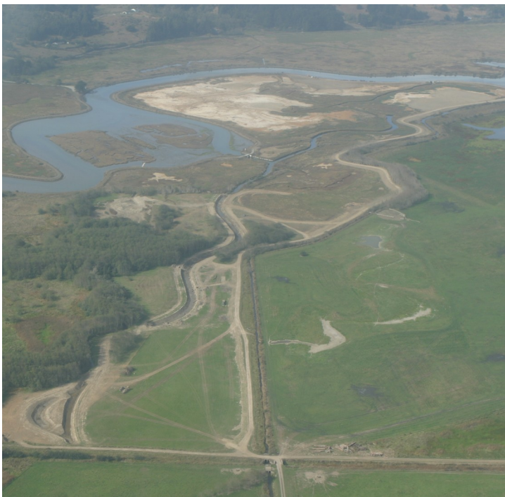
Figure 8. Aerial photograph depicting the newly constructed channel and side-channel pond in the foreground and subsided lands that were newly raised to support salt marsh in the background. We plan to continue channel excavation in 2011.
